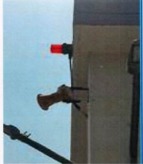
Alarm for Chlorine Leak Detection
