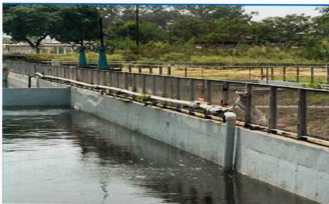
Chlorine Dosing Points in Chlorine Contact Tank
