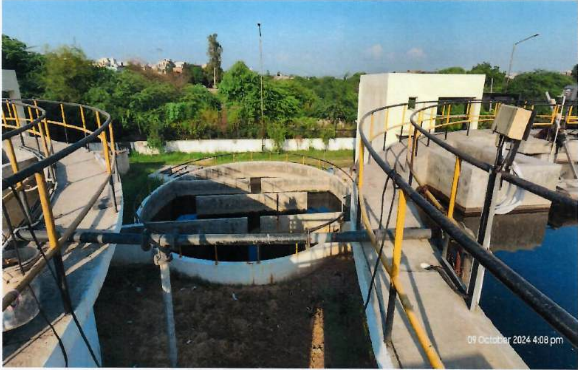
STP RAIPUR KALAN – II
