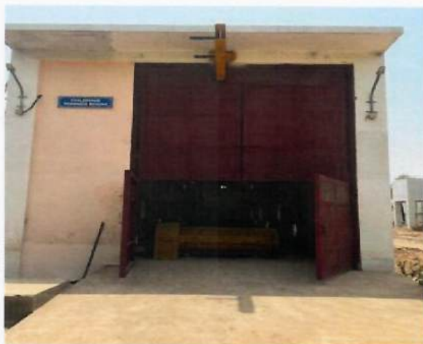
Chlorine Tonner with Manifold
