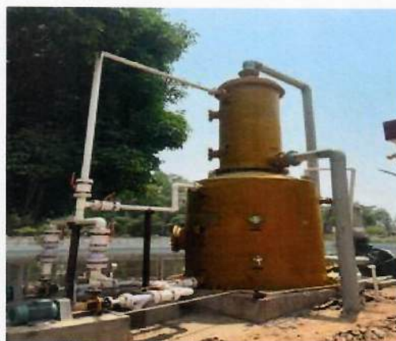
Chlorine Absorption System
